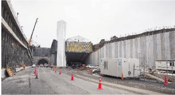
We should celebrate the opening of the nearly complete Waterview Connection, says Liam Dann, but there's still a lot of work to be done on Auckland's infrastructure. Picture / Nick Reed
